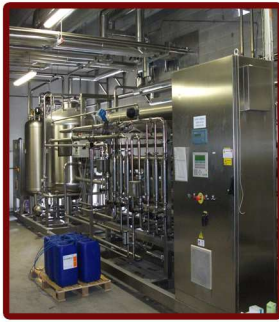
High Purified Water system , and distribution.
