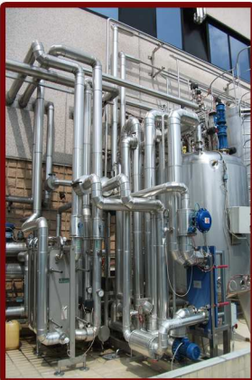
Media Preparation plant for BIOTECH
