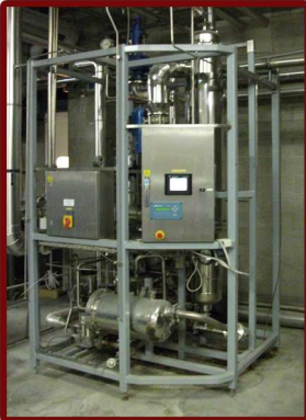
Clean steam and CF steam production system, and distribution
