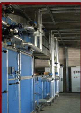
Air Handling Unit for special application, AHU for low humidity ratio.
