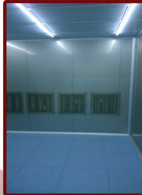
ISO6 Class cleanroom ,stainless steel wall, for powder mixing
